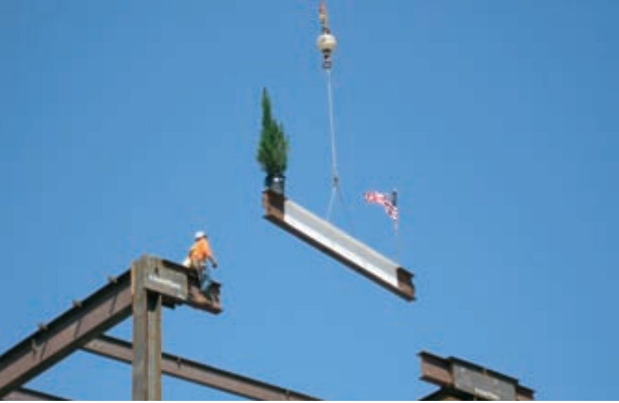
The final beam being placed at the top of the new fourth story.
